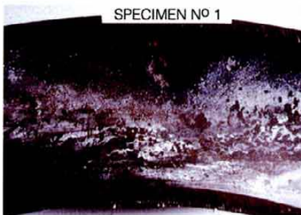
Failure of an austenitic steel heater tube caused by moisture condensing on the surface during shutdown.
